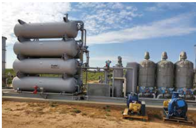
▲ Figure 7. This pressure-swing adsorption (PSA) system at a pig farm consists of four adsorptive vessels in series.
