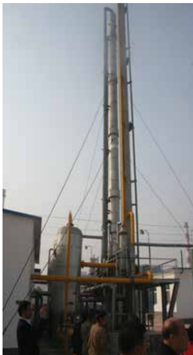
◀ Figure 9. This amine scrubber unit is installed at a digester site.
