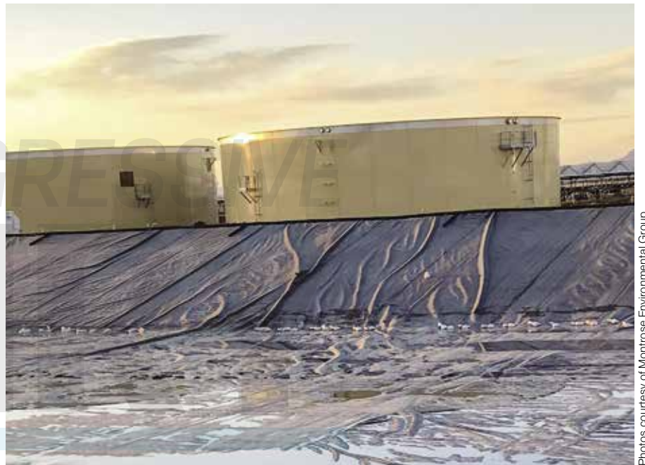
Two complete mix, 1.5-million-gallon digesters, with soft double membrane covers being built in Arizona.
