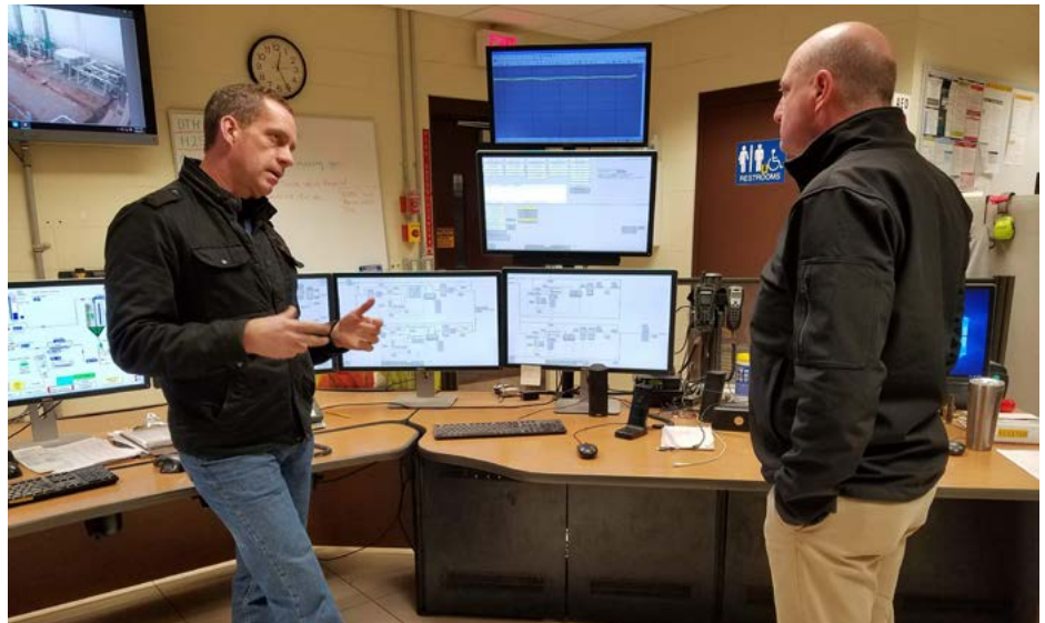
Klickitat PUD’s Kevin Ricks explains to NWPPA Executive Director Scott Corwin how they monitor levels, temperatures, and pressure in the control room, which is staffed 24/7.
